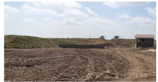
Pilot landfill in Thika – site clearance is made at the facility entrance, and the main gate and the management hut are under construction
