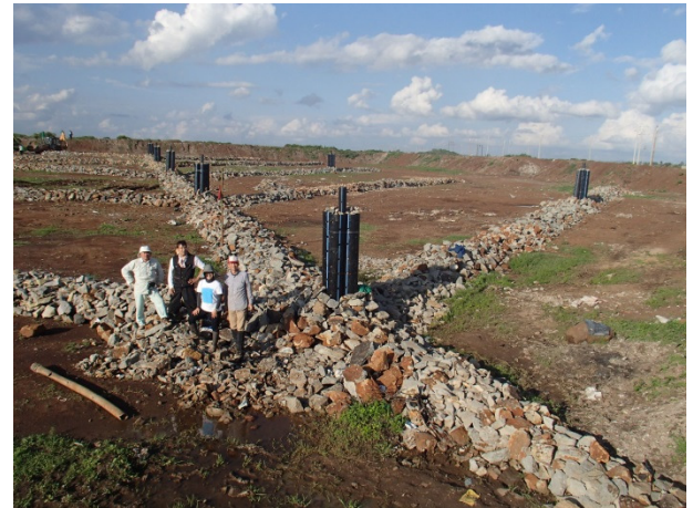
Completed landfill main body (1ha). The vertical venting pipes were installed during our last mission 完成した処分場本体(1ha)。鉛直ガス抜き管は我々の最後のミッションで設置
