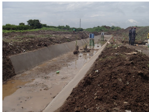
Overview of the leachate treatment pond. More water purification systems are better to be installed later
