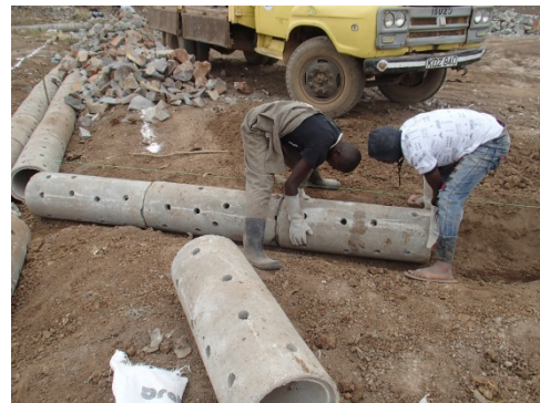
Perforated pipe installation: green string above the pipes is a leveling string / 穴あき管の敷設: 管の上の緑の糸が水糸
